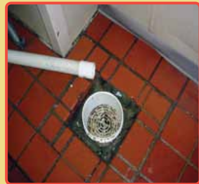
Figure 2.1. Pipe is not aligned properly with the drain causing standing water on the floor
