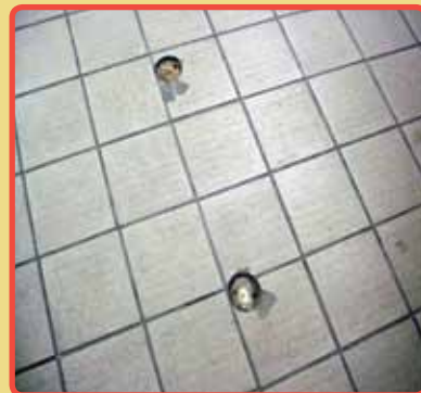
Figure 3.3. Tile floor where holes were not patched after something was removed
