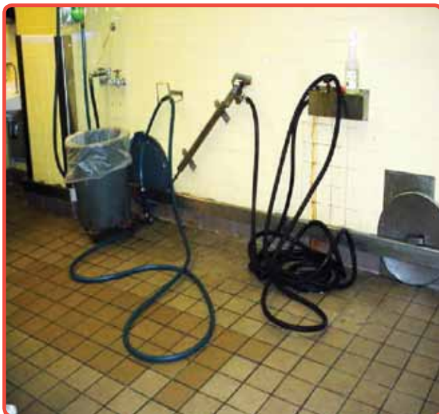
Figure 9.5. Uncoiled hose in a walkway
