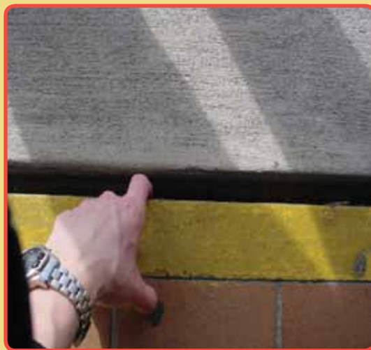
Figure 4.5. Large separation (greater than ½") in a walkway outside a hospital building
