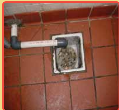
Figure 2.2. Drain is partially clogged with debris
