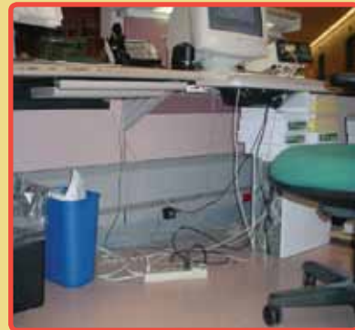
Figure 9.6. Loose cords at nursing workstation
