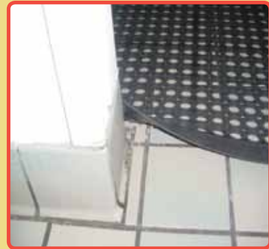
Figure 10.1. Edge of mat is not flat on the ground
