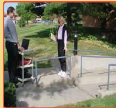
Figure 7.3. Discontinuous handrail too low for use by pedestrians
