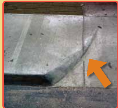
Figure 4.2. Area of sloped pavement that should be highlighted with Safety Yellow paint
